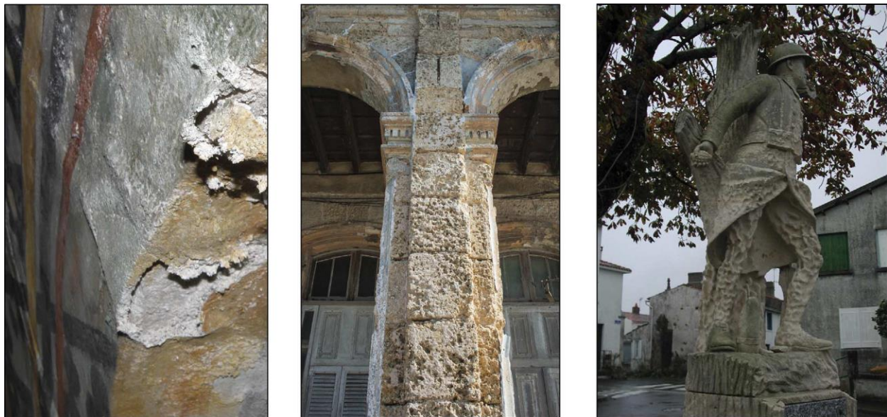
Figure 2.6. Examples of the devastating action exerted by salts on heritage masonry structures (Flatt et al. 2014)
