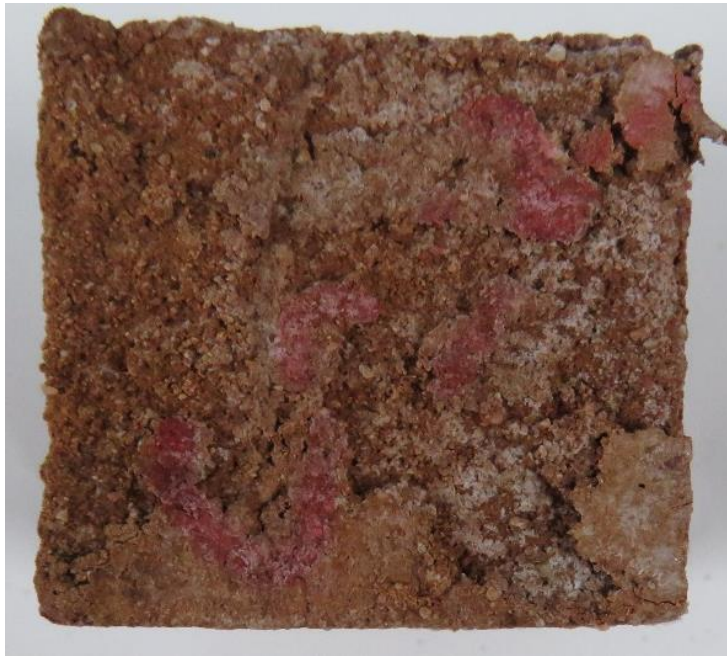
(b) The thin layer of the film gets cracked and removed for C2 treated with AS coating at 60 cycles
