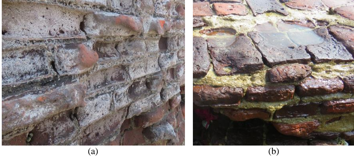
Figure 4.5. (a) Brick wall showing T1 bricks (b) T2 sample bricks which were partially immersed in seawater
