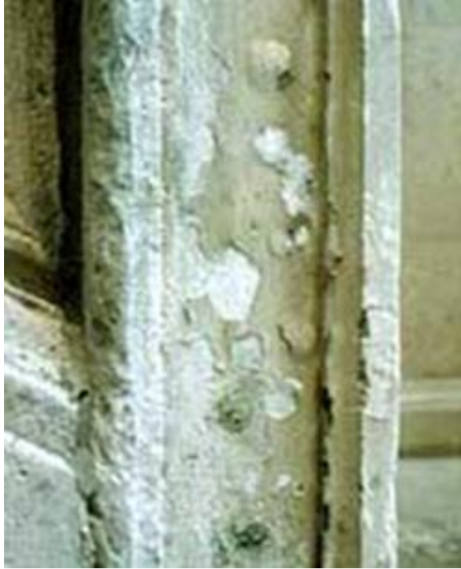
Figure 2.11. Protective coating damaging the stone substrate upon peeling (Mack and Grimmer 2000)
