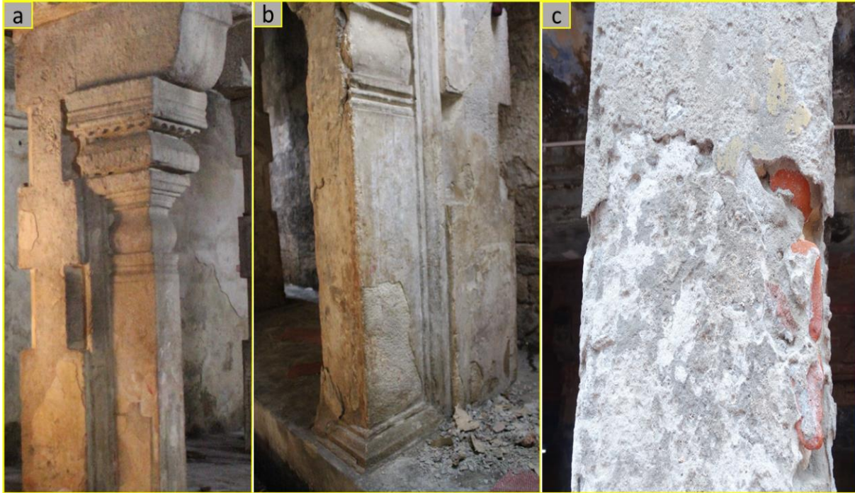
Figure 5.2. Coral stone columns showing damages of different degree (a) no damage (b) minor (spalling of plaster) (c) major (usage of improper incompatible brickbats leading to deterioration)
